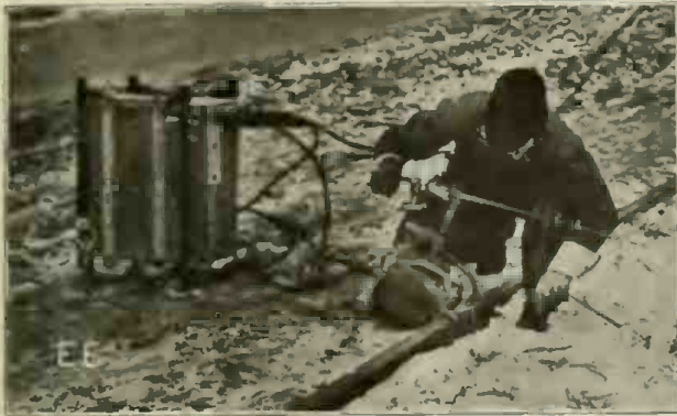
Welding Trolley Track Bonds With An Electric Furnace of Special Design. It Works Quickly and Is Portable. Time Per Weld Is About One Minute.
